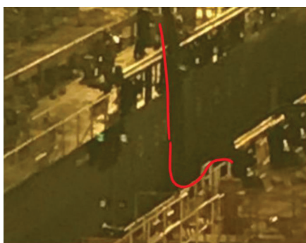
Incorrect lift causing U in hose
