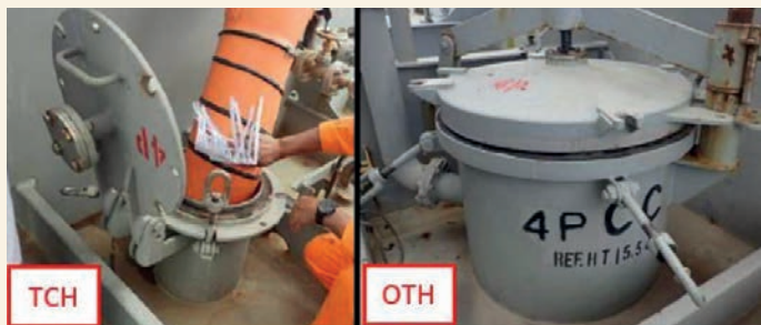
TCH Portable air chute connected to TCH
