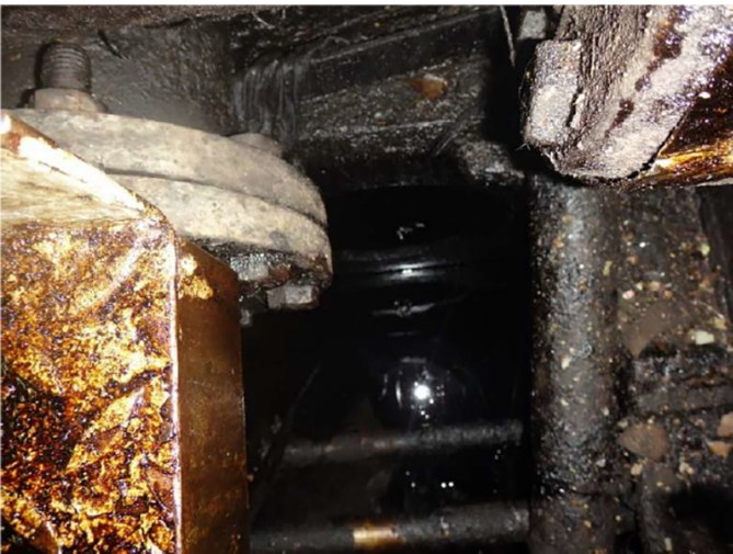
Oily bilges in the Engine Room
