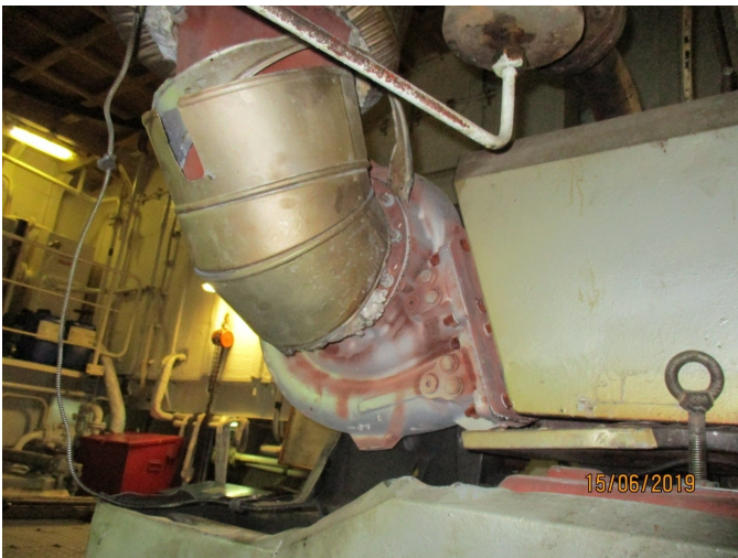
Damaged and missing insulation of the engine exhaust gas turbocharger and uptakes
