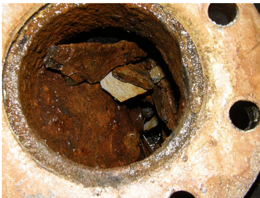
Rust and debris blocking this bilge well non-return valve allowed sea water to migrate into the hold during ballasting operations, causing cargo damage
