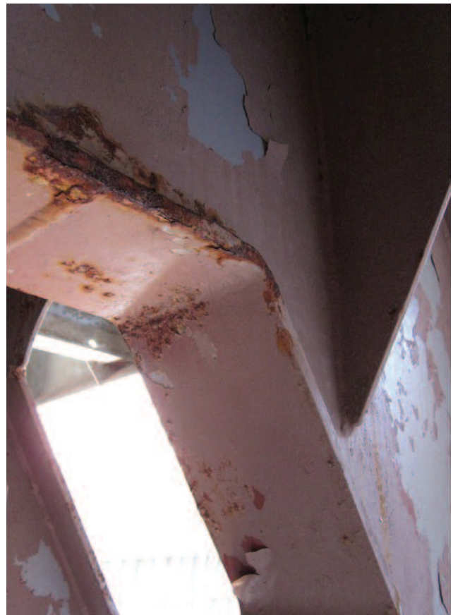
Flaking of paint coatings.
